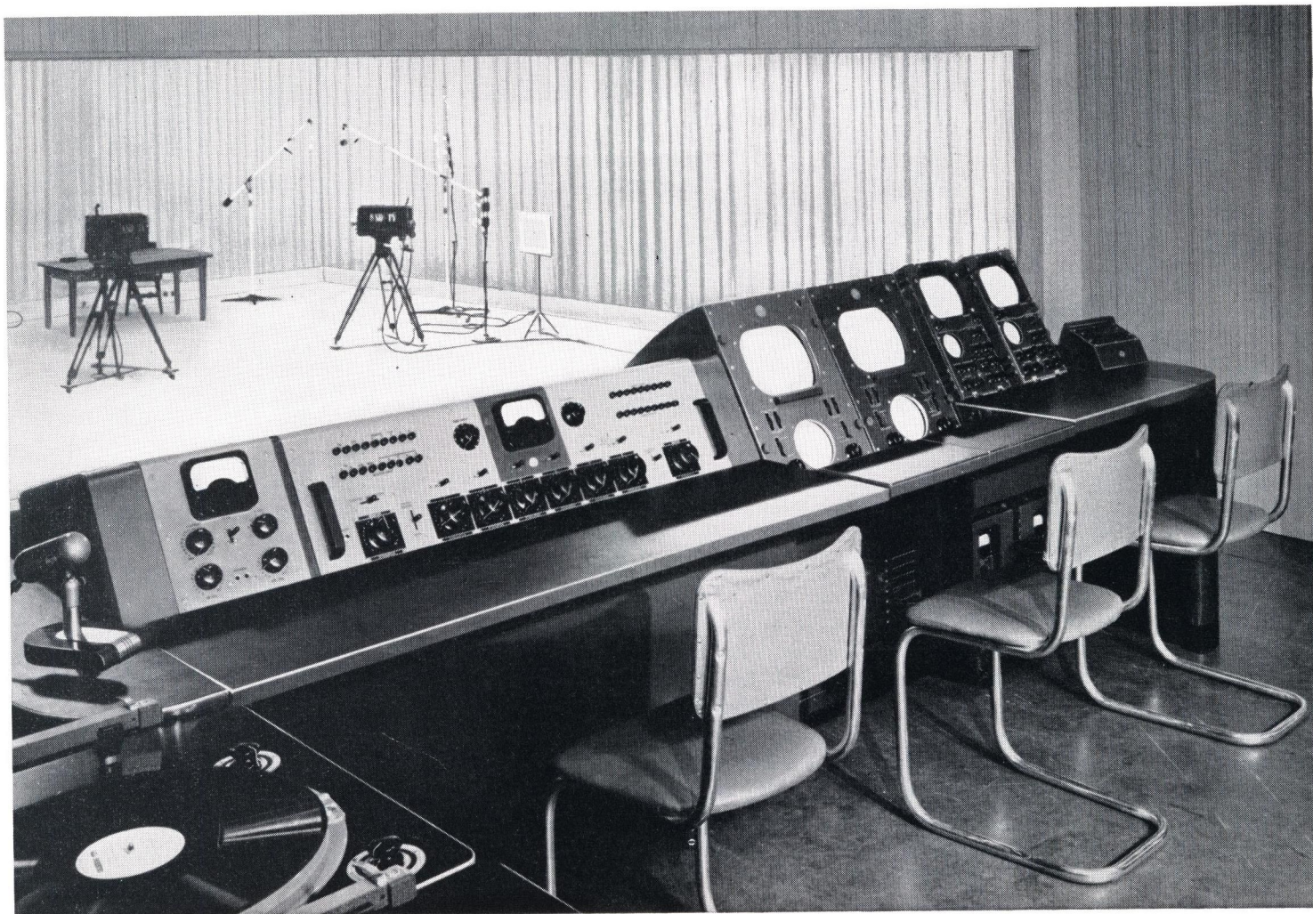
FIG. 16. (Below) Control Room for the Type B Small Station. This equipment layout utilizes the Type TS-10A Camera switching and lap-dissolving system, designed for studio control room use. Video units are identified in the block diagram, opposite page.
